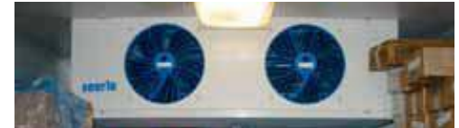
Above: Freezer room with defrosted evaporators and a well insulated drain
