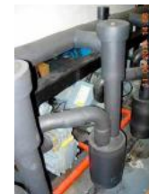
Above: Pipe Insulation
